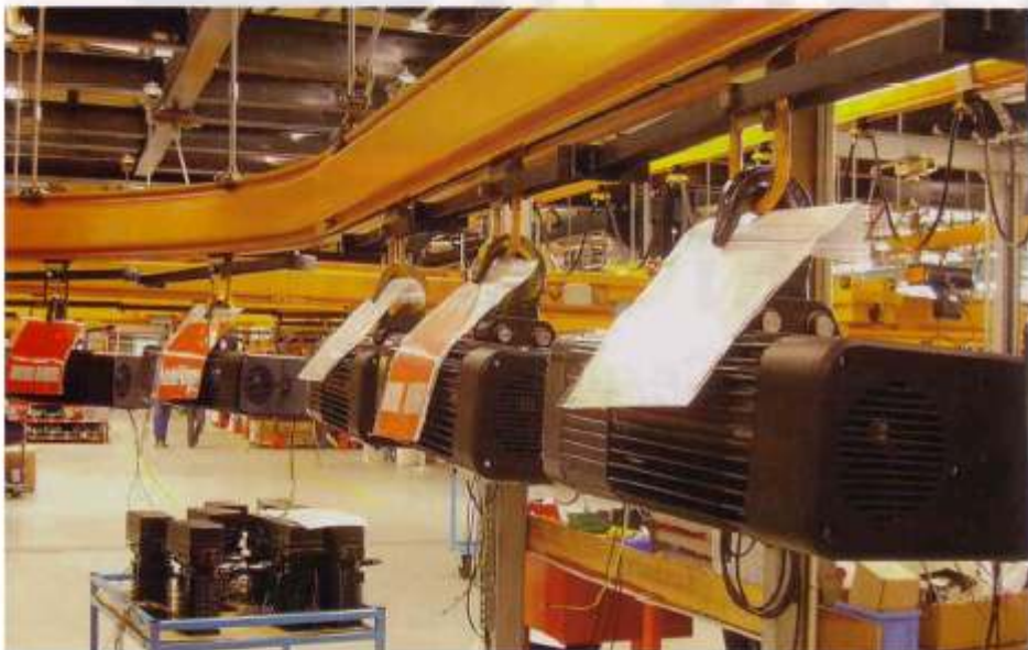
Small workstation cranes are not a big investment compared to overhead cranes. (Photo courtesy of Konecranes)
